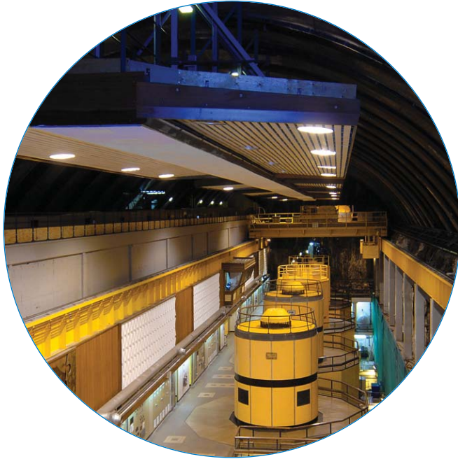
The station's machine hall, containing the four turbines, is the same size as a football pitch
