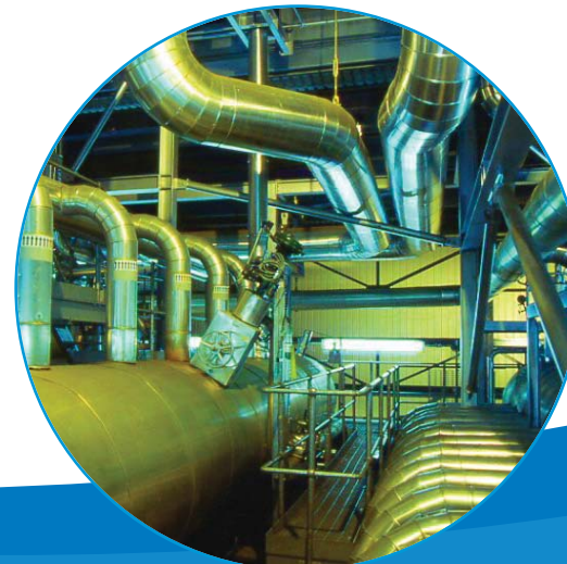
The Heat Recovery Steam Generator
