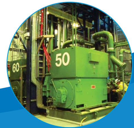
A boiler feed pump
