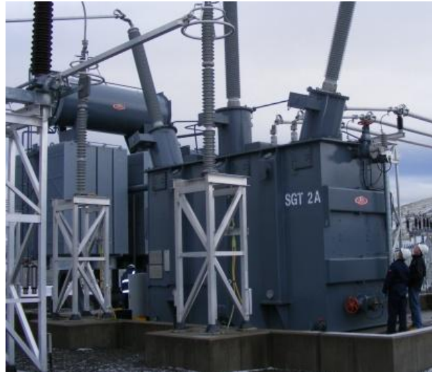
SGT 2A at Clyde North windfarm
